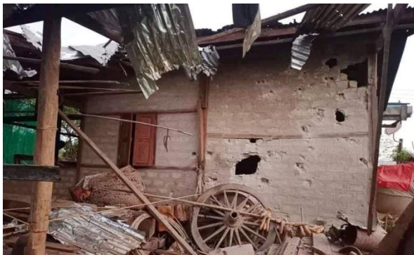
A house damaged by SAC shelling, Demawso
