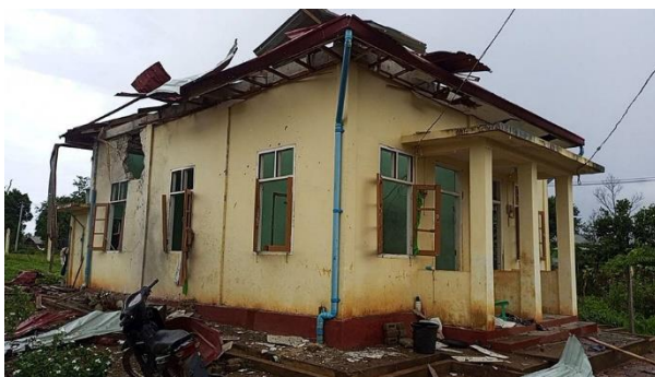
Building damaged by airstrikes in Loikaw
