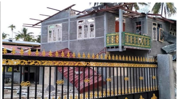
House damaged by SAC artillery shells in Lay Pho Gyi village, Loikaw township
